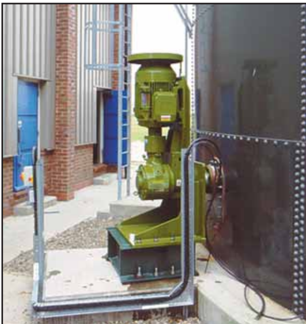
Lightnin Plenty LRES side entry mixer with independent mounting on glassed steel sludge tank.
