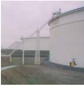
Swivel angle belt driven mixers installed in a crude oil terminal in Netherlands
